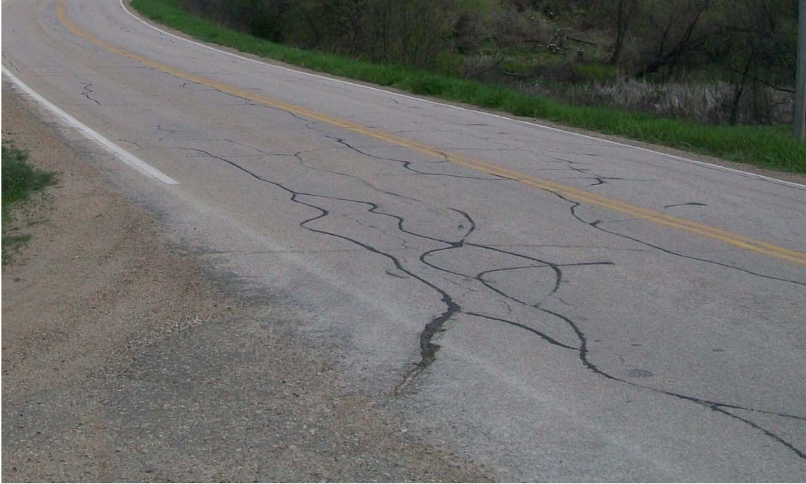
Crack Sealing is excessive due to asphalt pavement age
