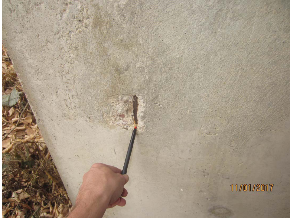
Exposed reinforcement on north end of east abutment
