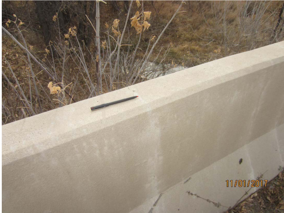
Cracks on guardrail
