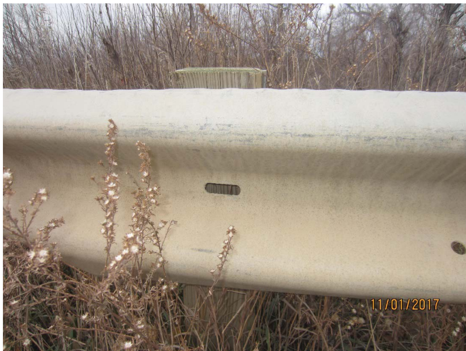
Missing bolt in guardrail
