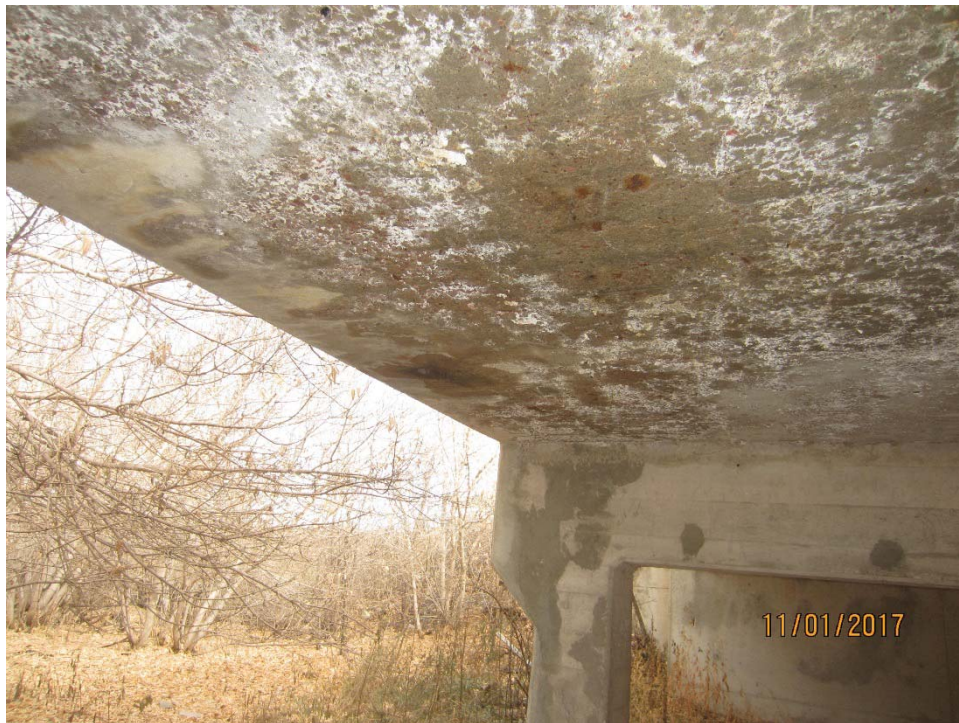
Bottom of slab water damage from drains
