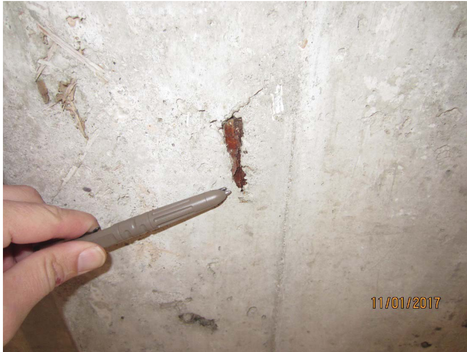
Hole in Beam
