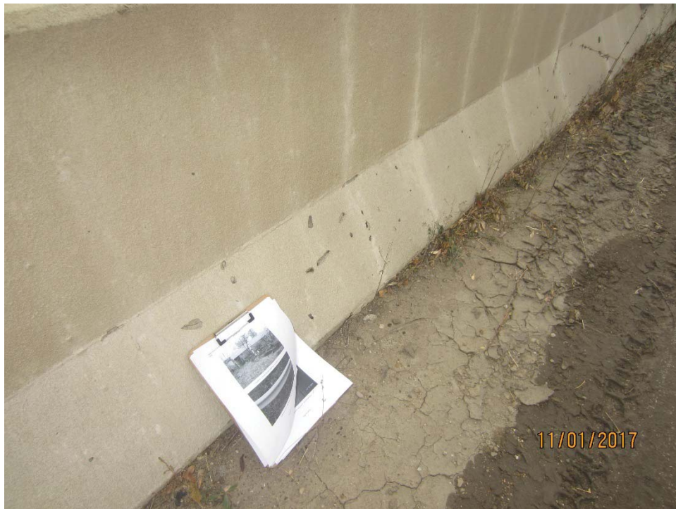
Surface finish peeling on bridge rail
