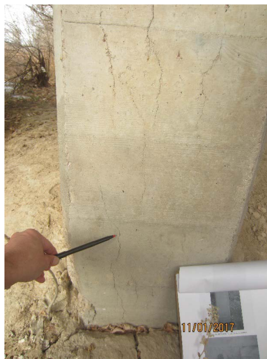
Pier cap cracking
