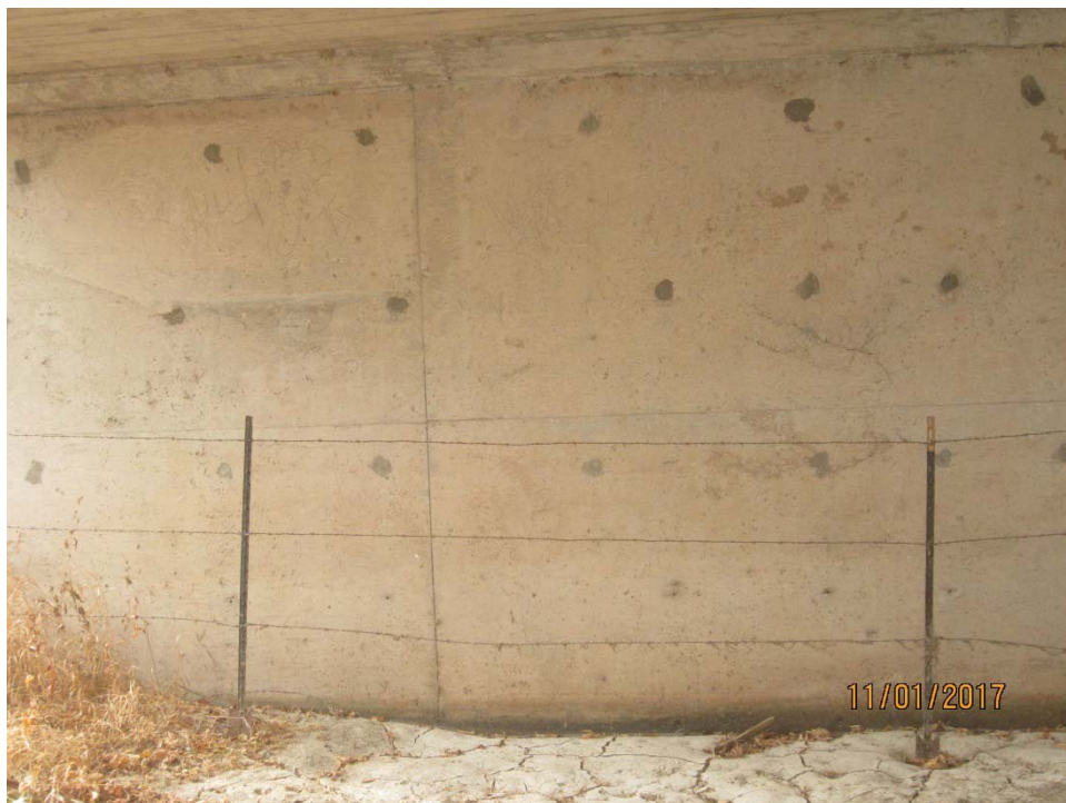
Cracking on S abutment
