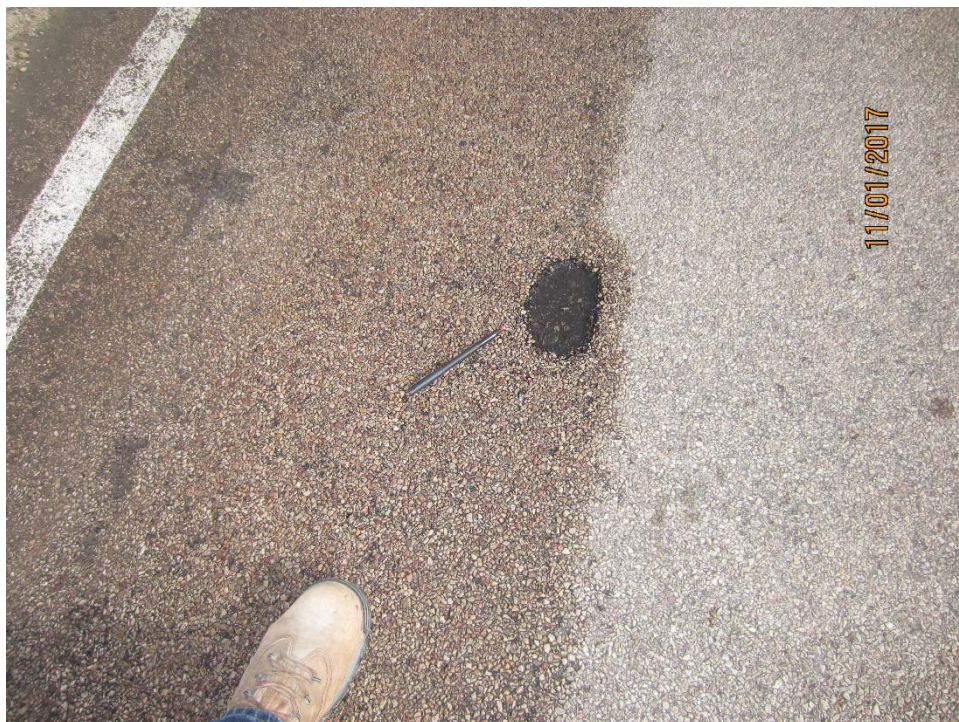
Asphalt overlay failing.
