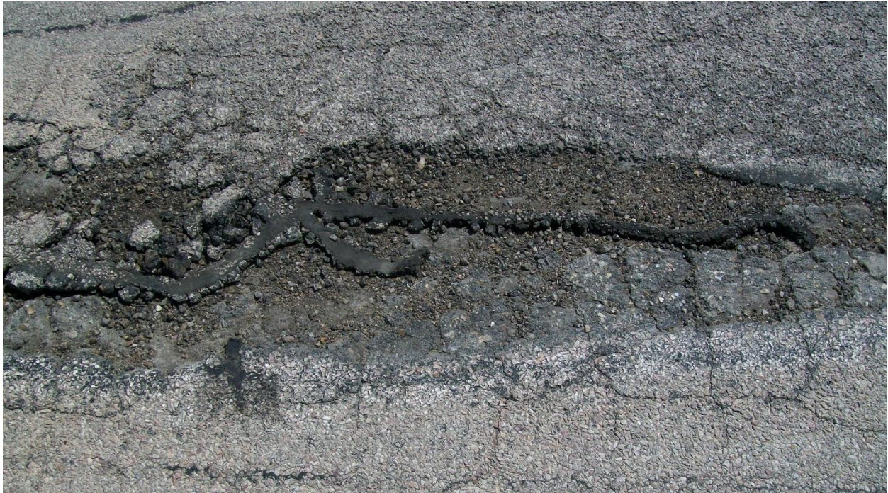
Figure 4.5: Alligator Cracking on BIA 2
