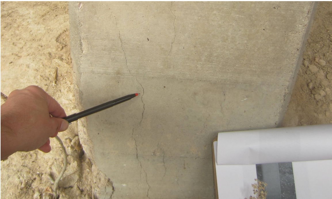
Potato Creek Bridge – Column Cracking and Spalling
