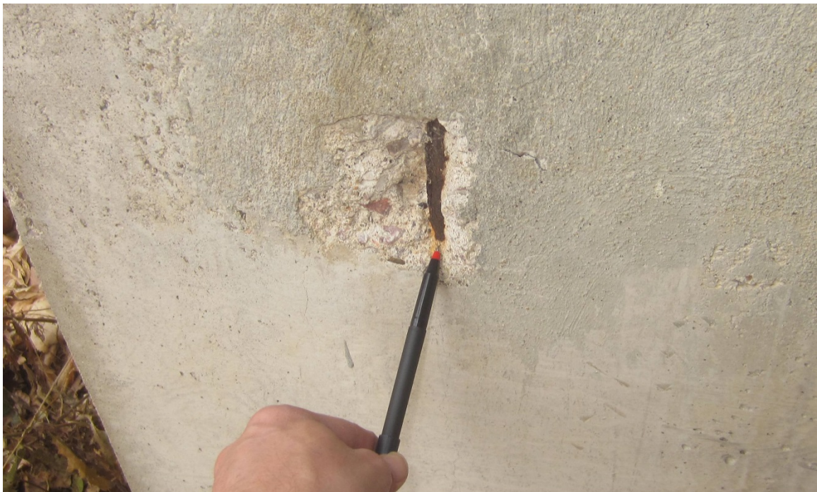
Potato Creek Bridge – Exposed Steel Reinforcement in Column
