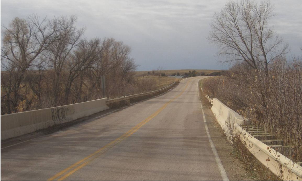
BIA 2 – looking west – inadequate sight distance
