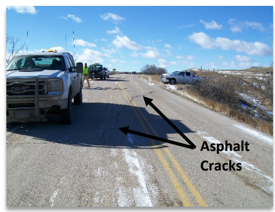
Roadway west of Potato Creek Bridge is exhibiting an embankment slide and being monitored
