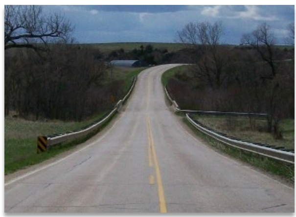
Potato Creek Bridge is 75-80 years old, for photos and descriptions of the aging structure's issues www.oglalasioux.raisegrant.net
