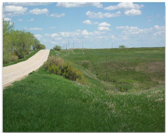
BIA 2 road geometry is 75-80 years old and pavement is 40 years old, for photos and descriptions of the aging structure's issues www.oglalasioux.raisegrant.net
